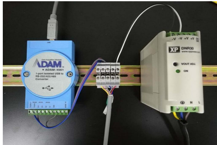
Figure 3.1 Power Supply and 485 converter
